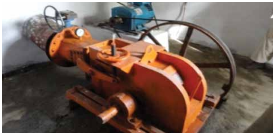
Turbine of the Power House Near Jodbah
